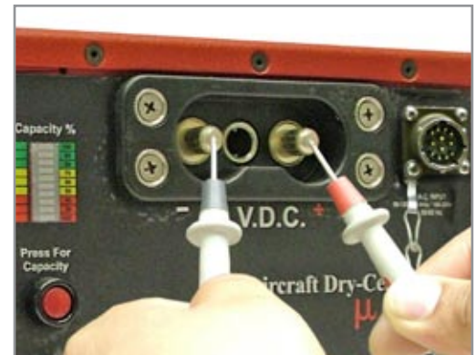
Figure 3.8.3 – Testing DC Receptacle
