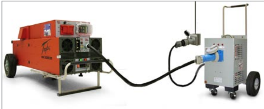
Figure 4.4.1 Transformer connected to GPU
