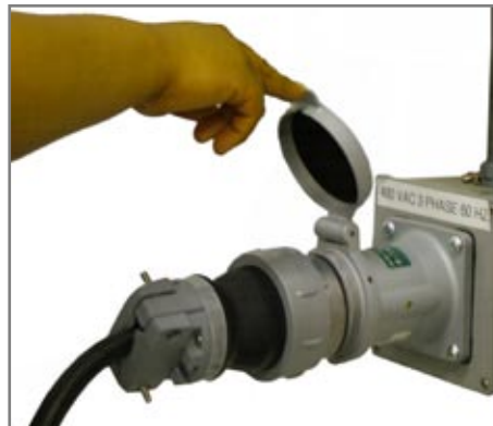
Figure 2.7.2 480 VAC cable plugged in.
