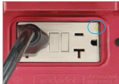
Figure 6.3.4 – 60Hz AC Power Outlet "ON" (green LED illuminated (outlined in blue))
