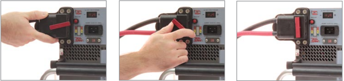
Figure 3.11.1 Attaching DC Power Cable to TI3000 GPU-24-INV-1800
